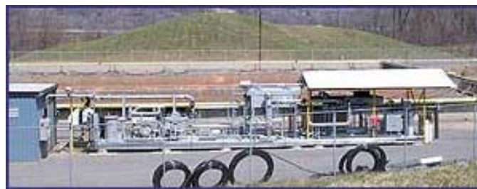
Figure b - Wayne Township Landfill Gas System
