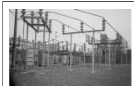
Figure 3. Substation located near the town of Vashon
